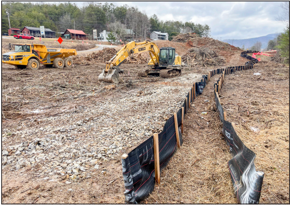
Phase II of the project continues between Earl Shelton Road in Union County and Sampson Road in Towns County. Photo by Shawn Jarrard
